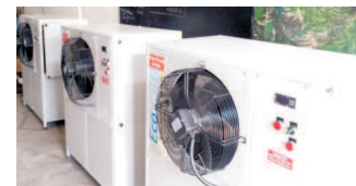
Heat Pump [HP]
